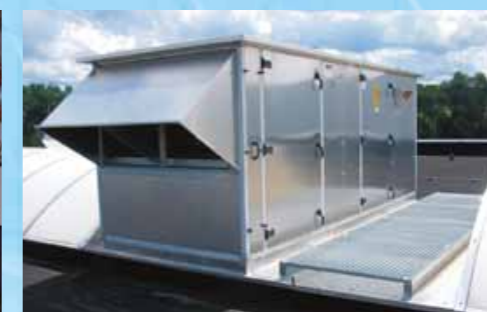
Ventilation system on the roof of a building
