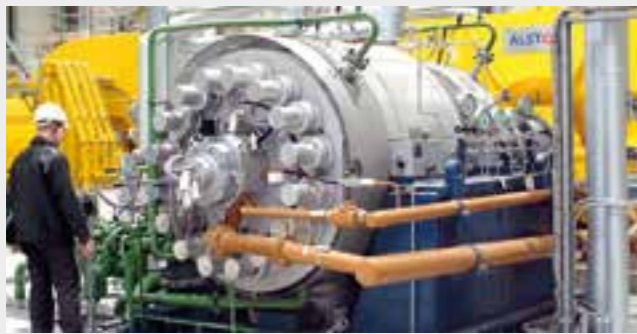
A centrifugal pump at a power plant
