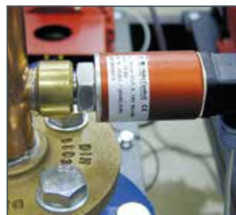
Each pump has an inlet and outlet above pressure sensors
