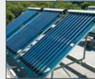
Solar thermal energy
