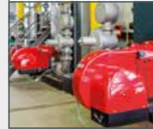
Oil, gas or wood-fired boiler
